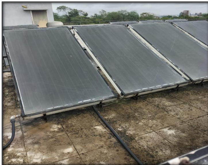
Photograph of Roof Top Solar Water Thermal Water Heating System:
